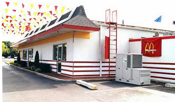
Plug Power small stationary PEM fuel cell outside a McDonald's outlet in the USA. (Courtesy of Plug Power)
